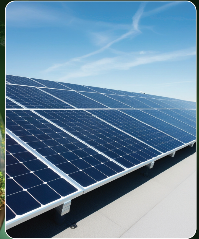
5 KW Solar Panel for each villa
